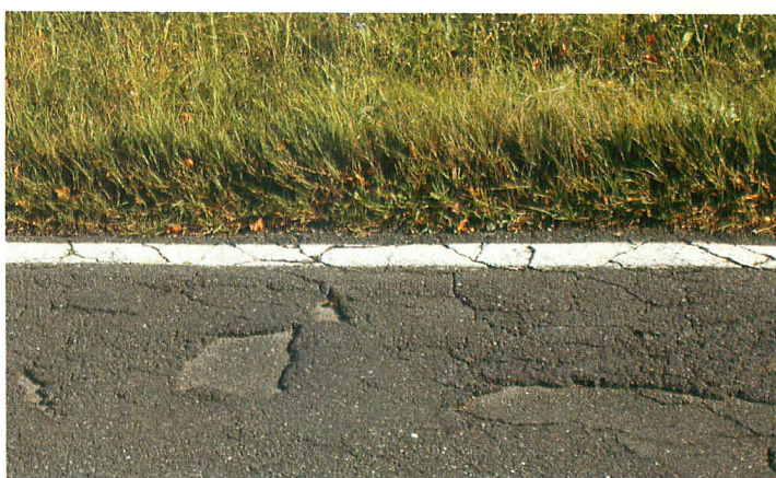
➤ Cost cutting at the wrong end – this type of disrepair puts motorcyclists in danger.
