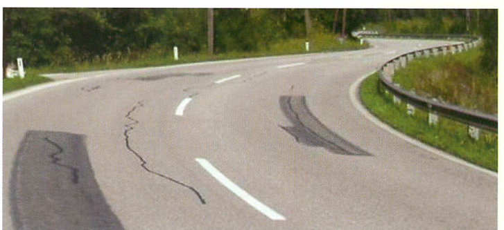
➤ Serious flaws in the road pavement: patches of varying grip, lane ruts and “patchwork” repair.
