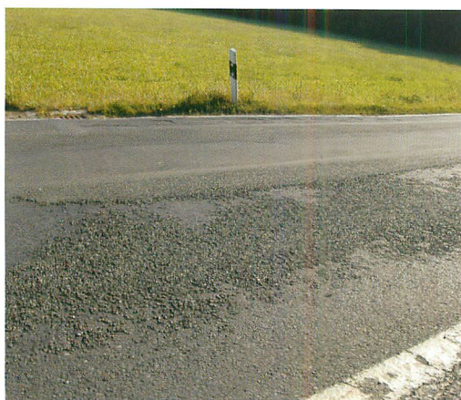
➤ Dangerous state of disrepair – no shoulder profiling; poor condition of road markings.
