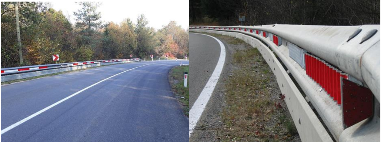
Figures 27 and 28: Increased visibility of bend at night: red-white strips for guiding on bends in combination with SGR with additional motorcyclist protection and double-sided 3312 signs for guiding traffic on bends (Source: U. Brumec)
