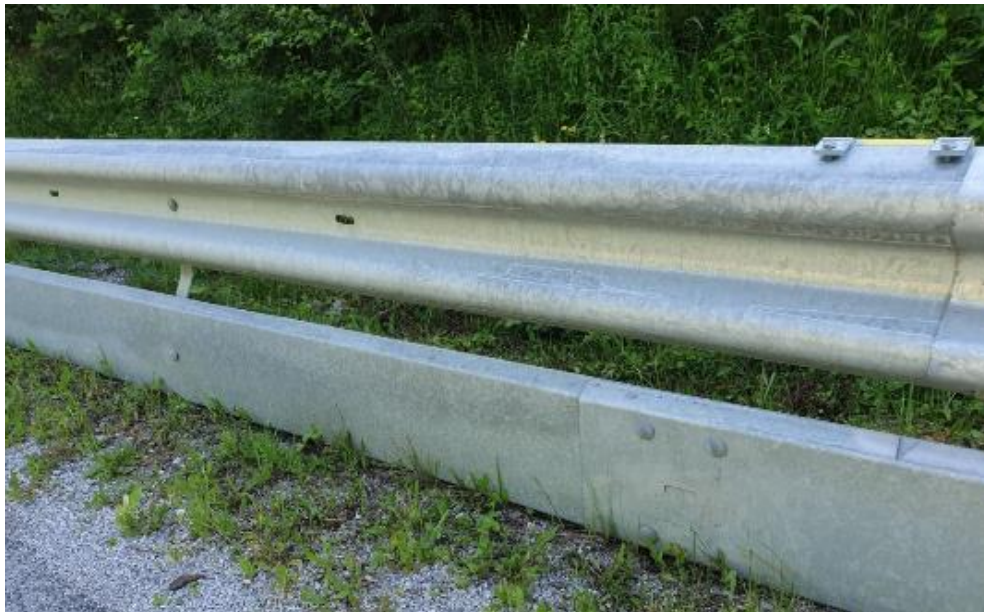
Figure 3: Proper installation of additional protection for motorcyclists on steel guard rail (source: T. Tollazzi).
