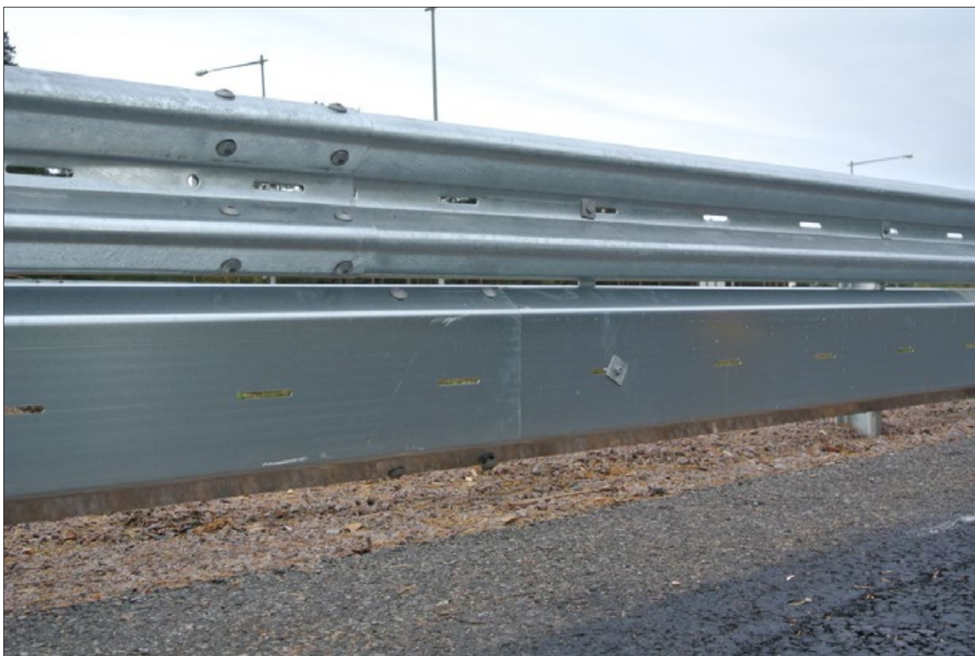
Picture 3. W-profile barrier with MPS, installed on an exit of E4 outside Gävle 2014.
