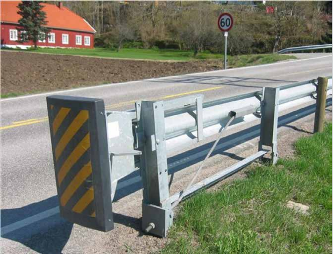
Picture 26 - Guardrail terminals present sharp edges and a low contact surface, face traffic directly and are located very close to the roadway. Fitting them with a protective cover reduce the risk of injury on impact.
