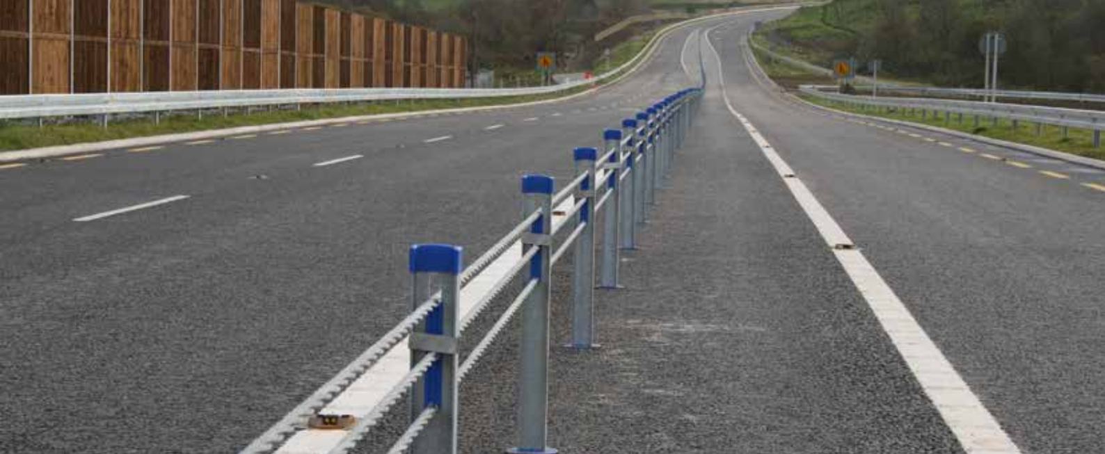
Picture 7 - Wire Rope Barrier
