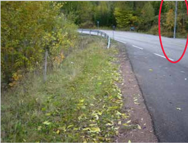
Picture 21 - Problem : lamp post in hazard zone
